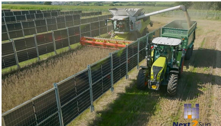
Next2Sun's 5.2 MW Agrivoltaic vertical PV installation, featuring Huasun's Kunlun series HJT module, exceeds power generation expectations by 12%, noted the project manager. (Photo Credit: Huasun)
